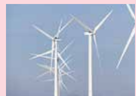
Wind Power Generators
