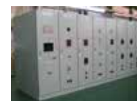
High Voltage Receiving Panels Sanyu Electric Corporation
