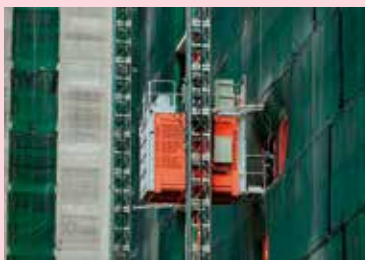
Construction Elevators & Lifts
