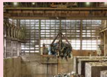
Waste Disposal Plants
